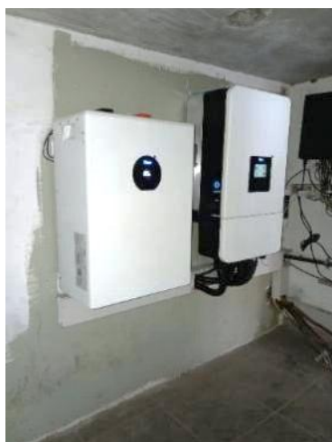
Power storage backup
