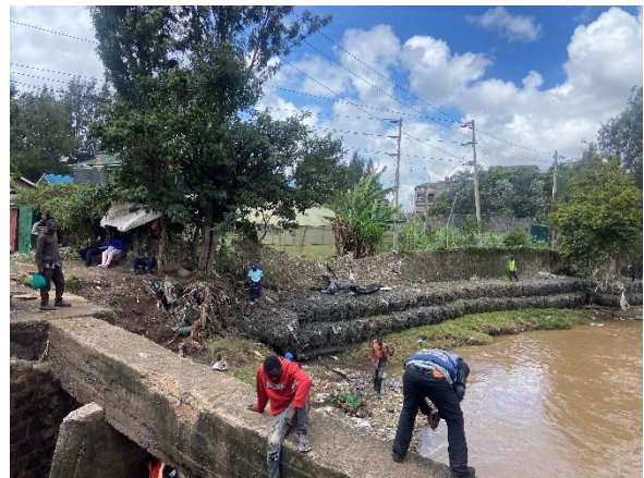
Fence collapsed, and gabions exposed
