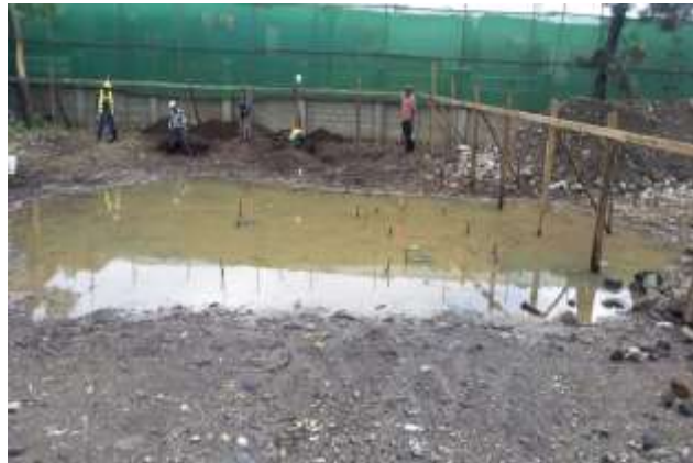
After heavy rains
