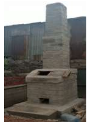
Incinerator ready for use
